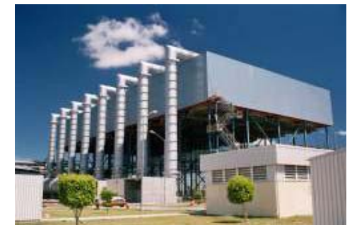
Dry Cooling System
