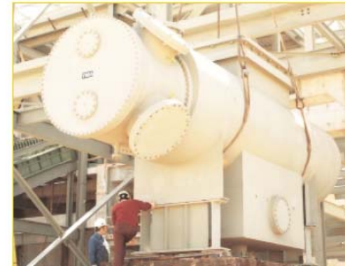
Steam Surface Condenser
