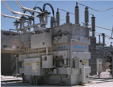
Medium Power Transformer
