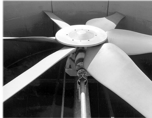
Air Flow Components
