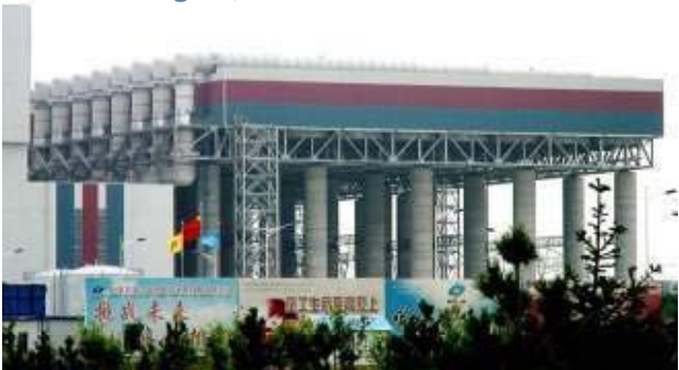
SPX cooling system in Zenglan, China
