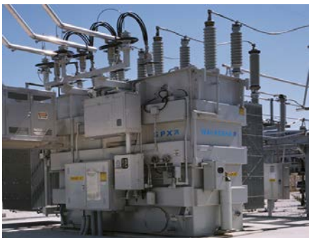
Medium Power Transformer
