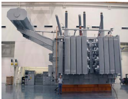
High Voltage Transformer
