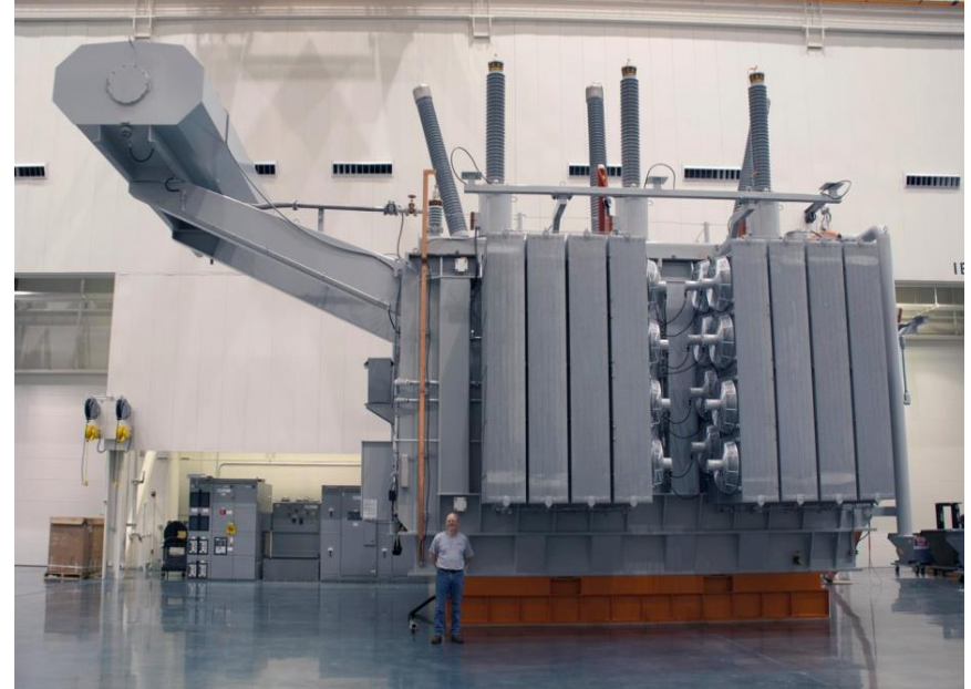
Large Power (High Voltage) Transformer
