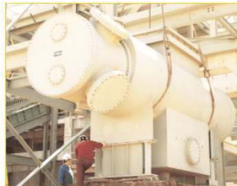
Steam Surface Condenser
