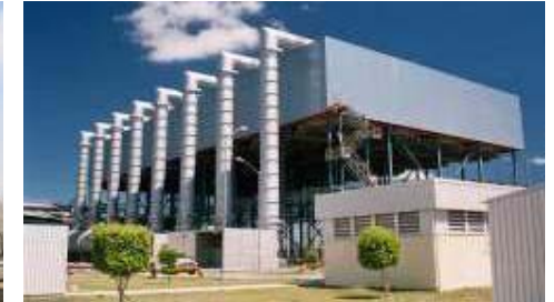
Dry Cooling System
