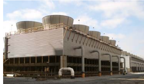
Evaporative Cooling System
