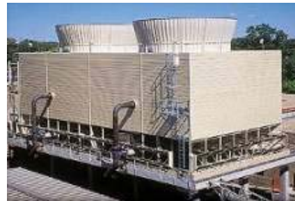
Wet Cooling System
