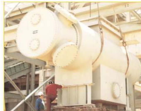
Steam Surface Condenser
