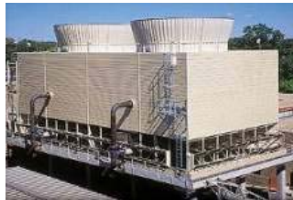
Wet Cooling System
