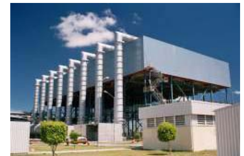
Dry Cooling System
