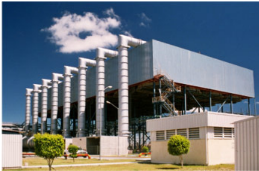
Natural Gas Power Plant in Mexico
