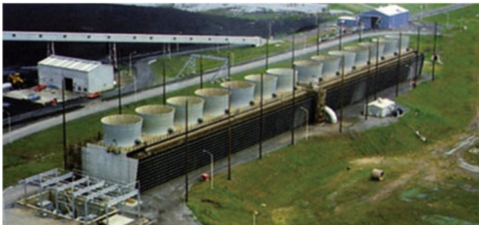
Coal-Fired Power Plant in the United States
