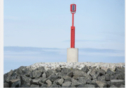
Marine Obstruction Lighting
