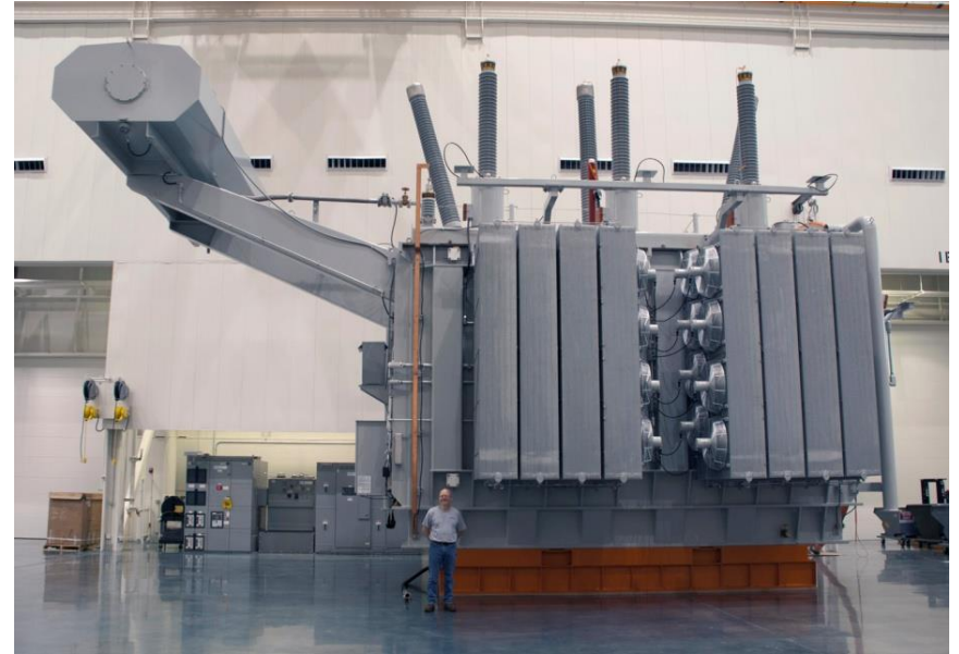
Large Power (High Voltage) Transformer
