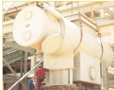
Steam Surface Condenser
