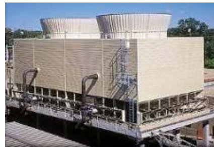
Wet Cooling System
